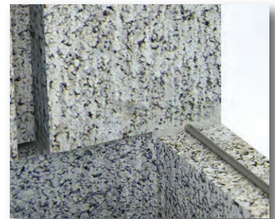
Figure 4. Heavy-duty, 3/16-inch-diameter wire can leave inadequate room for proper mortar coverage. Both the top and bottom of wire could be in direct contact with masonry unit (no mortar coverage).
